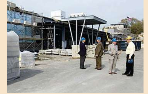
Construction in progress on the new hospital addition at 350 South Huntington Ave., 2005.
