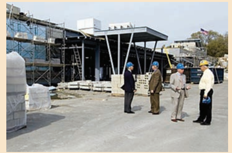
Construction in progress on the new hospital addition at 350 South Huntington Ave., 2005.
